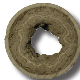
Cooling water pipes after less than one year's operation without filtration.
